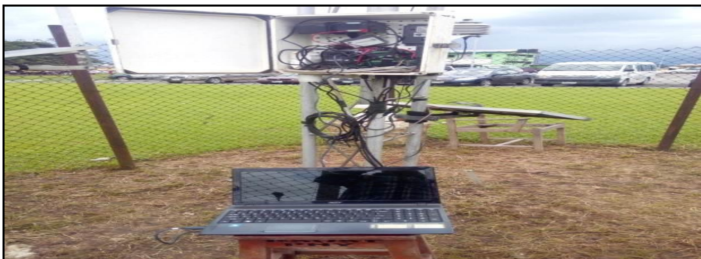
Figure 6: A view showing the connection between a laptop and the Electronics Box in the weather station
